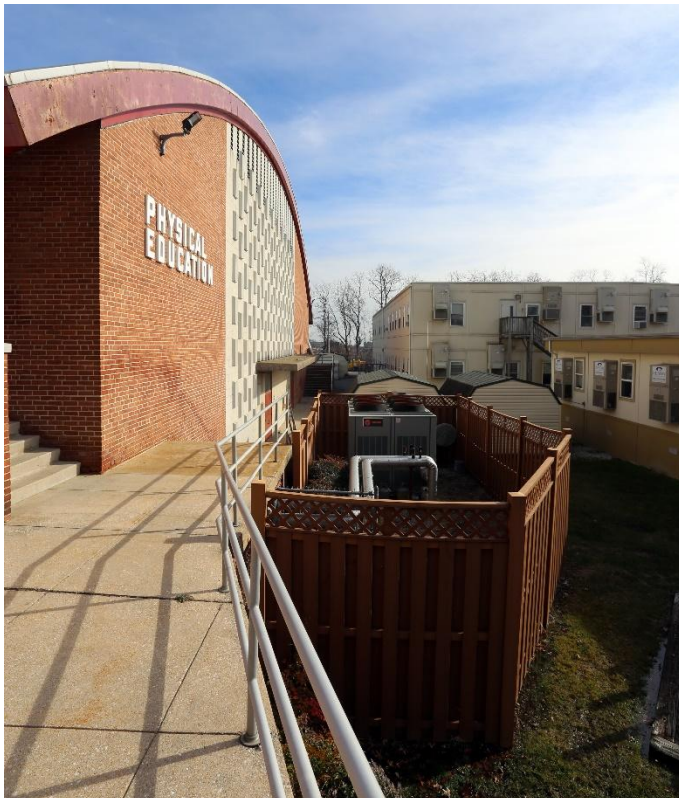
Figure 4-35 – Mechanical clutter and encroachment at the front of the gymnasium
