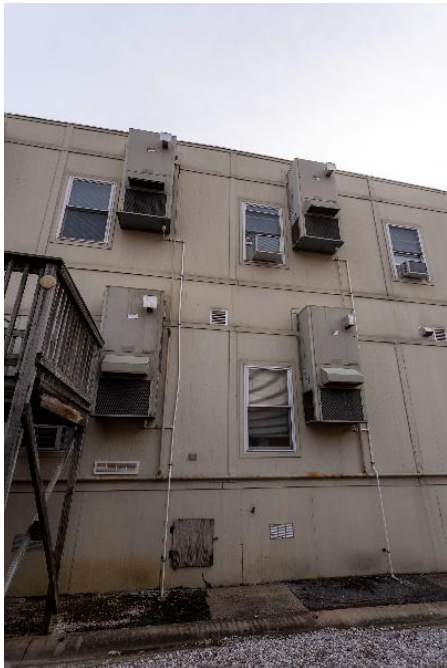
Figure 4-59 - Typical PTAC units
