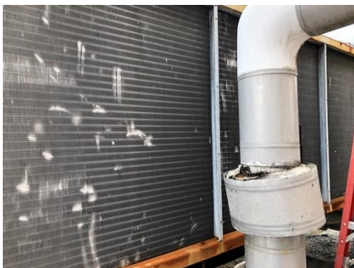
Figure 4-65 - Existing Air Cooled Chiller
