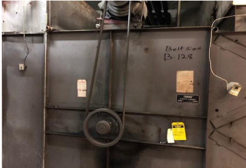
Figure 4-31 - Existing Dual Duct AHU
