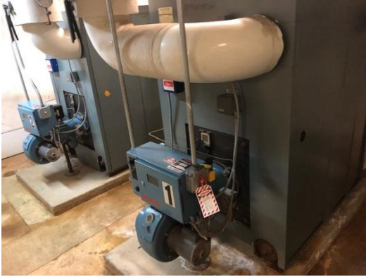
Figure 4-36 - Cast Iron Boilers
