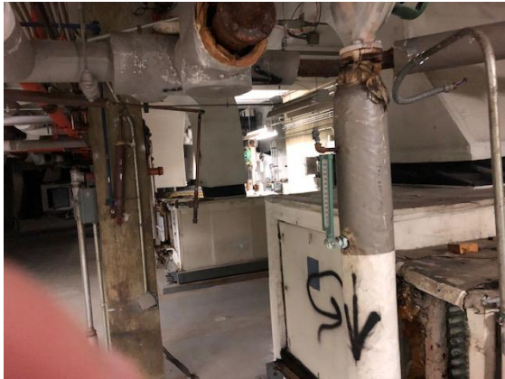
Figure 4-66 - Abandoned AHU in Basement Mechanical Room
