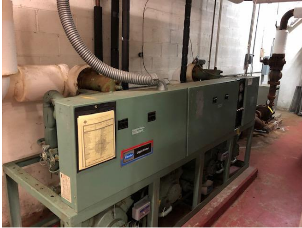
Figure 4-27- Chiller and Condensing Unit
