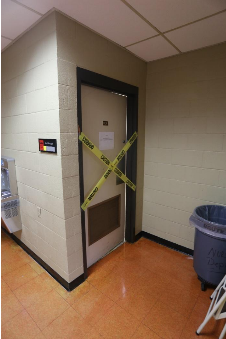
Figure 4-40 – Toilet out of service
