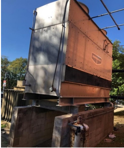
Figure 4-41 - Building Cooling Tower
