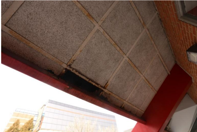
Figure 4-34 – Damaged Tectum and framing at gym roof overhang
