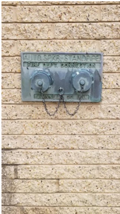
Figure 4-67 - Fire Department Connection for sprinkler system.
