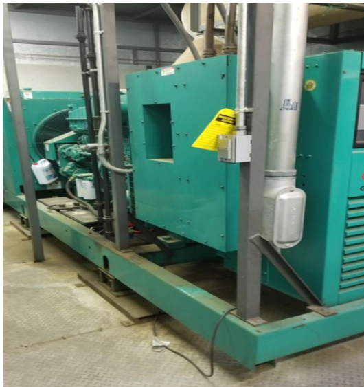
Figure 4-51 - Diesel-engine drive Emergency Generator
