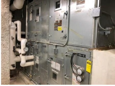
Figure 4-18 VAV Air Handler, Typical for Each Wing
