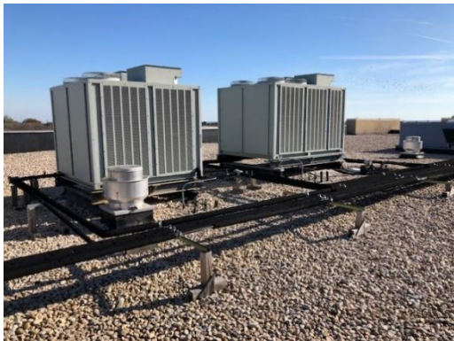
Figure 4-74 - Rooftop Condensers, One Per AHU.
