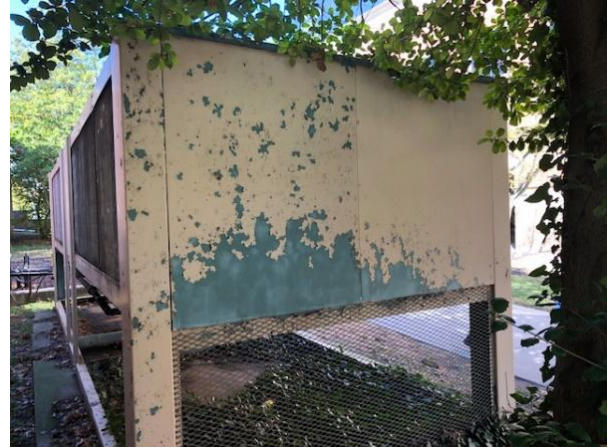
Figure 4-28- Chiller and Condensing Unit
