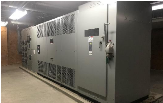
Figure 4-20 Switchgear with Transformer and 480V feeder outputs for the entire Administration Building
