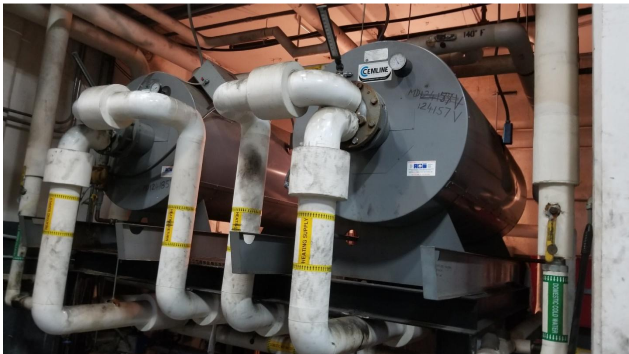
Figure 4-19B Domestic water heaters in boiler rooms
