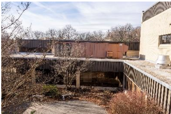
Figure 4-81 - Rooftop Unit and Exhaust Fan
