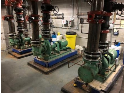
Figure 4-15 Condenser Water Pumps
