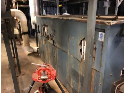
Figure 4-48 - Cast Iron Boilers Serving Life Sciences Building
