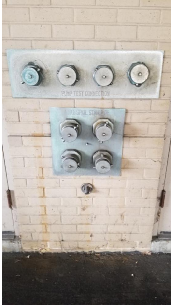
Figure 4-50 - Fire pump test heads and Fire Department Connection
